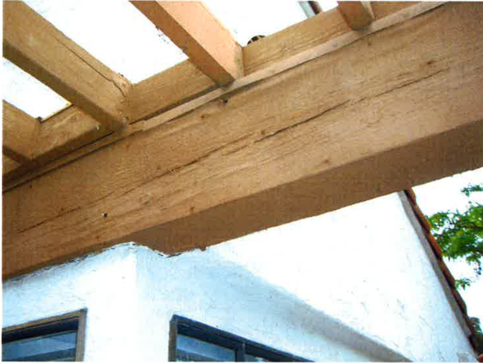
Figure 58: Termite and dry rot damage
