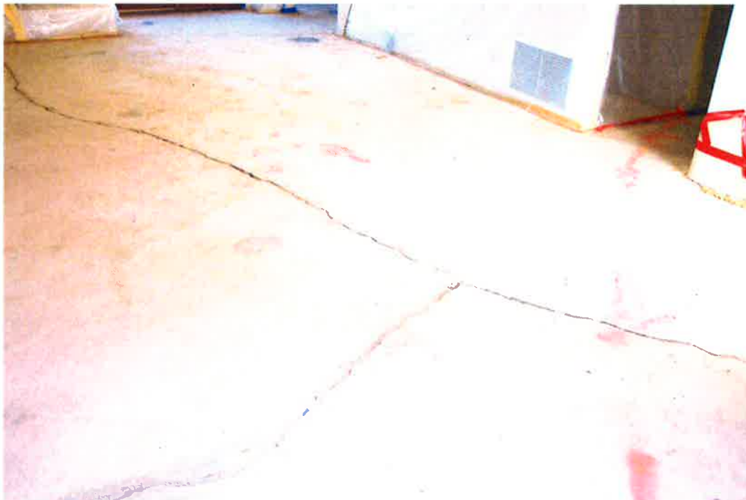
Figure 4: Slab cracking and damage as a result of ground settling
