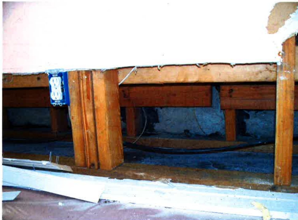
Figure 69 - View from interior of wall under pot shelf showing deteriorated building paper from sustained moisture conditions and pot shelf leakage
