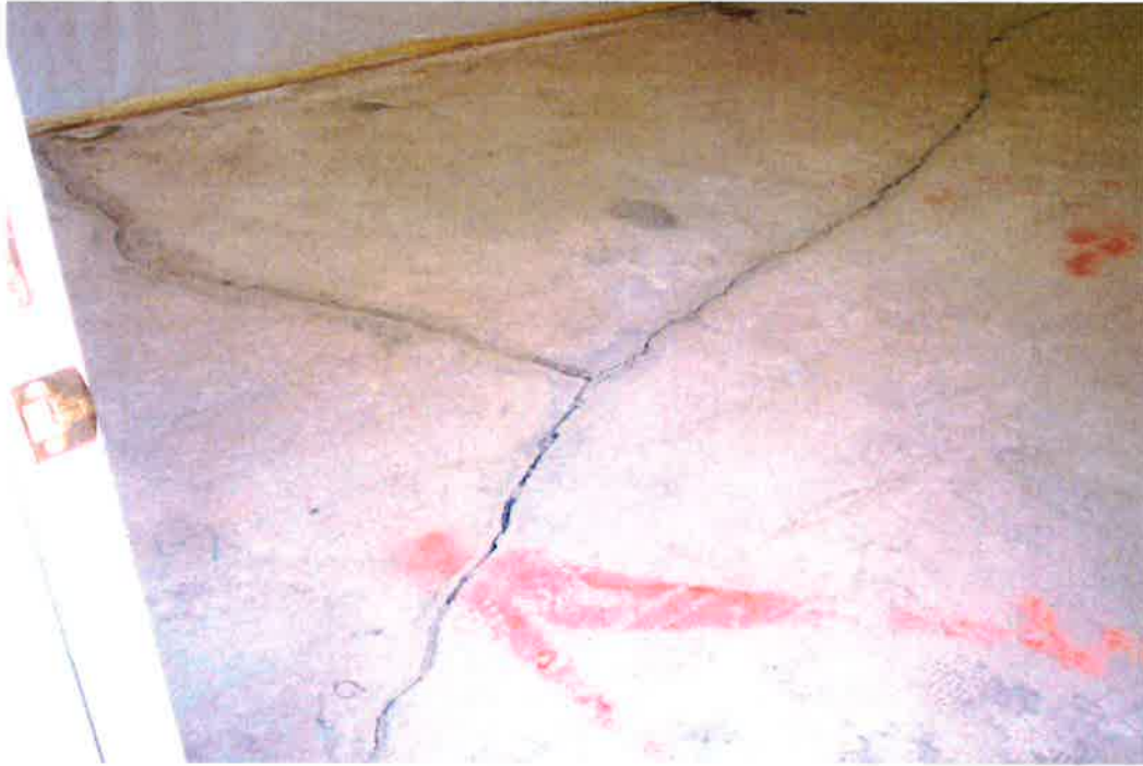
Figure 3: Slab cracking and damage as a result of ground settling
