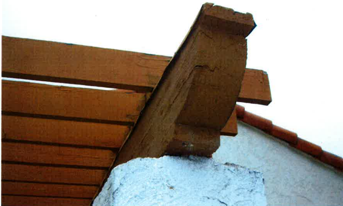
Figure 61: Termite and dry rot damage
