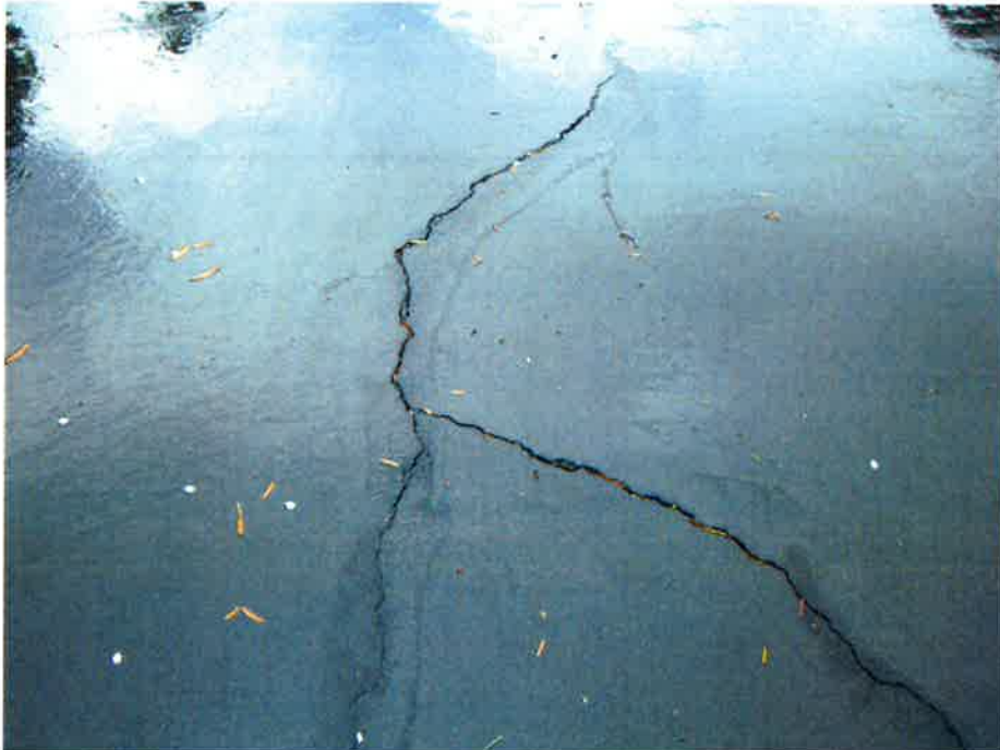
Figure 77: Cracks allow moisture, causing additional damage
