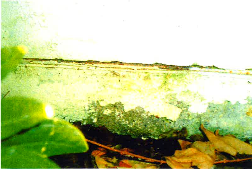
Figure 37: Failed stucco; Spalled footing (from moisture)
