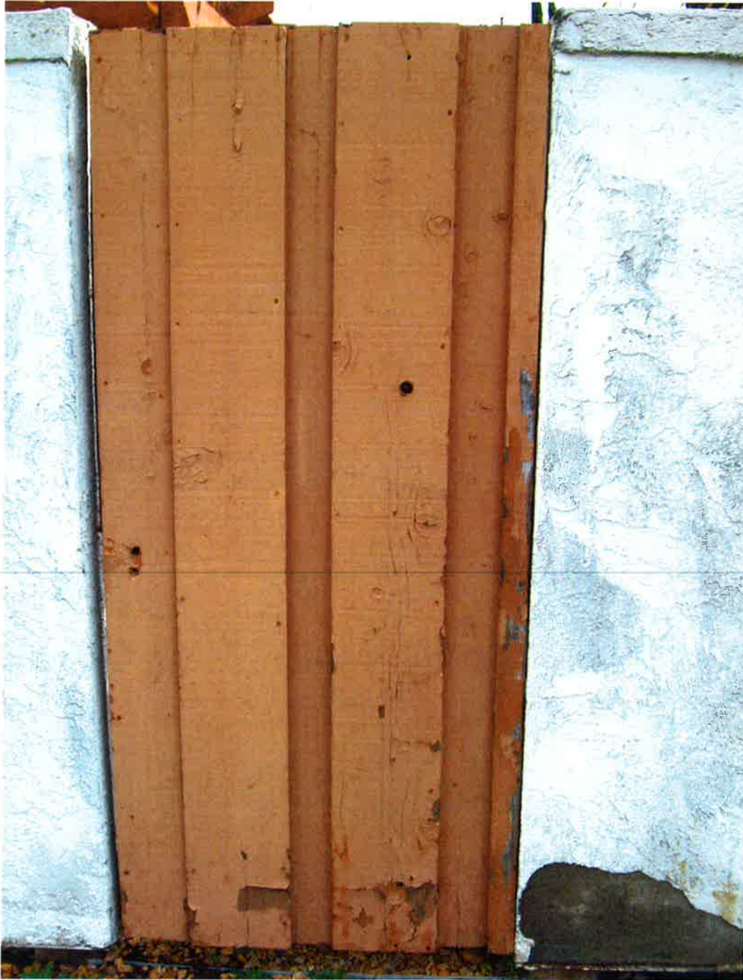
Figure 71: Door paint condition
