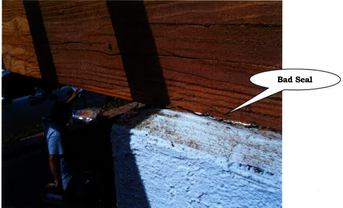
Figure 56 Bad seal between pop-out and trellis beam above front elevation windows
