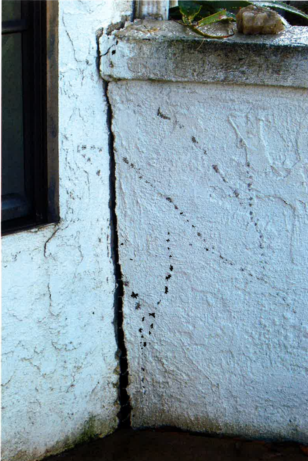
Figure 24: Rotted post resulting in wall settling
