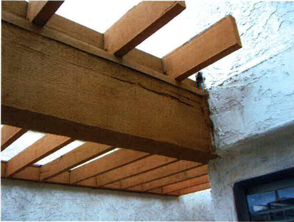
Figure 62: Deterioration of supporting beam into Pop-out beam above windows
