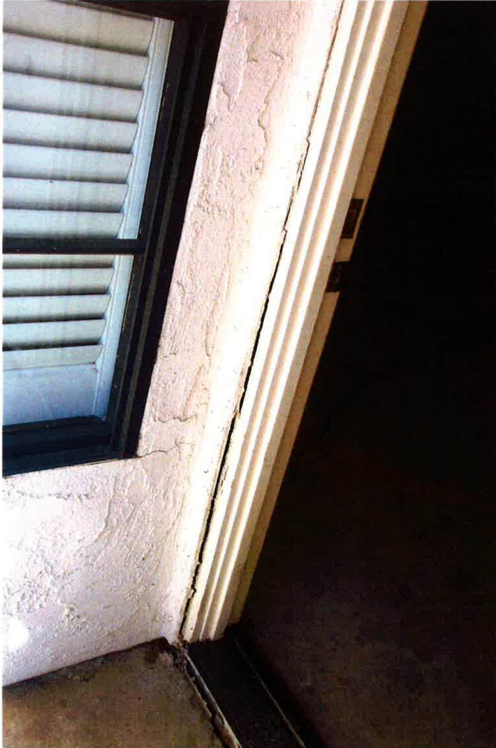
Figure 14: Wall separation from Pressure Grouting re-leveling of building
