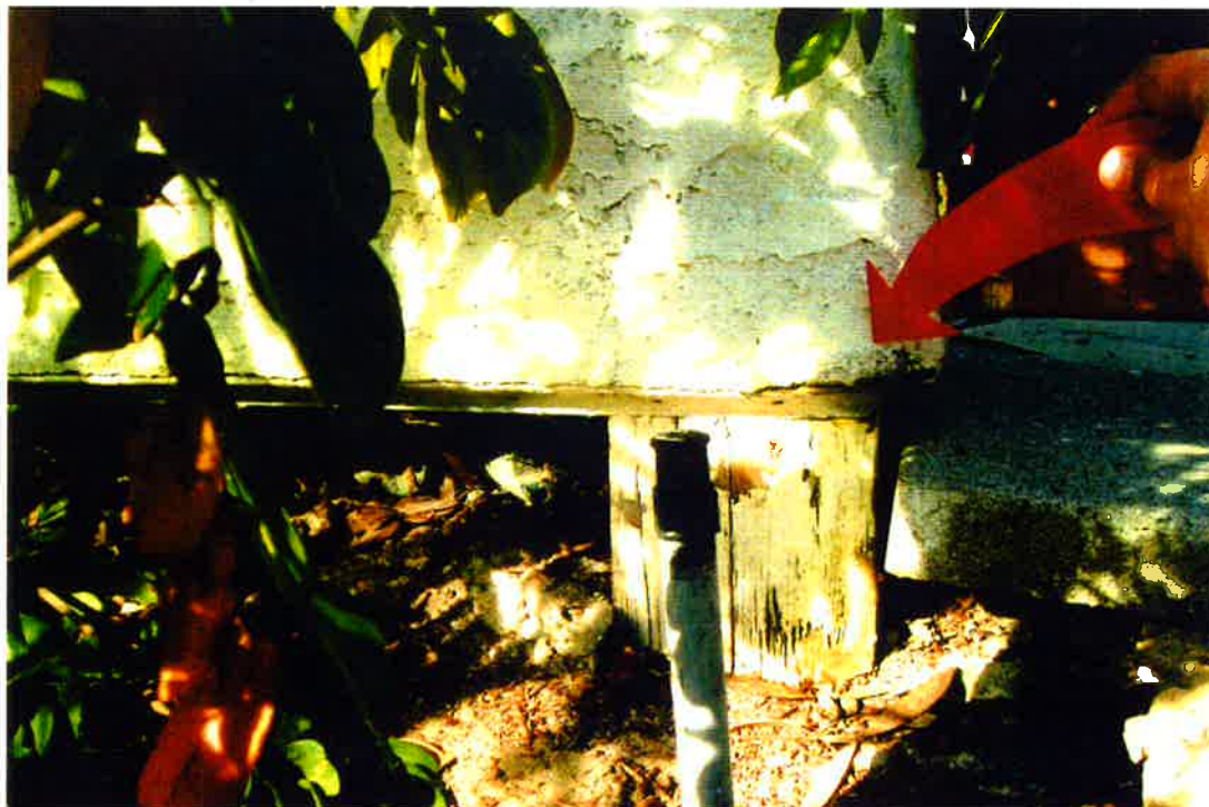
Figure 28: Stucco fence - rotten post
