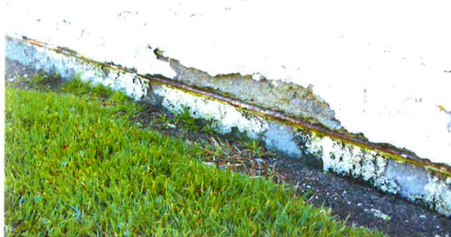
Figure 26: Stucco failure; weep screed
