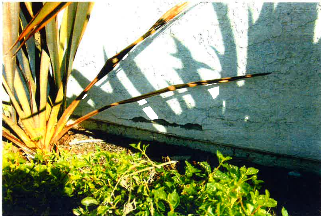
Figure 32: Stucco failure - sustained moisture
