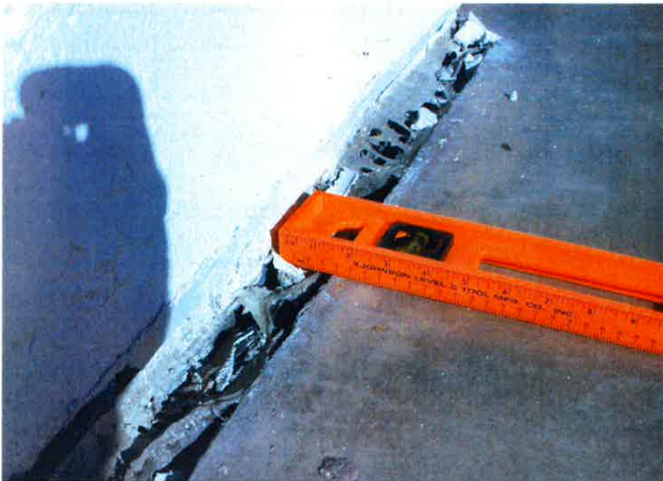
Figure 6: Patio sliding away from wall as slope moves
