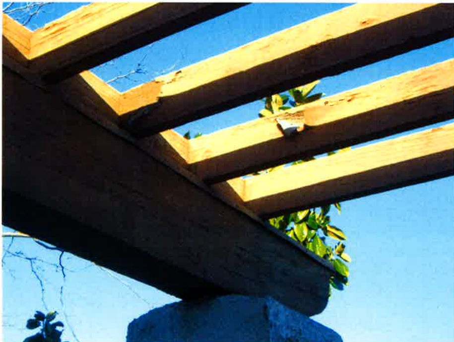
Figure 65: Termite and dry rot damage
