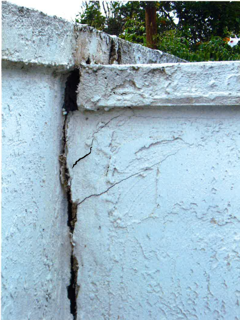
Figure 23: Rotted post resulting in wall settling
