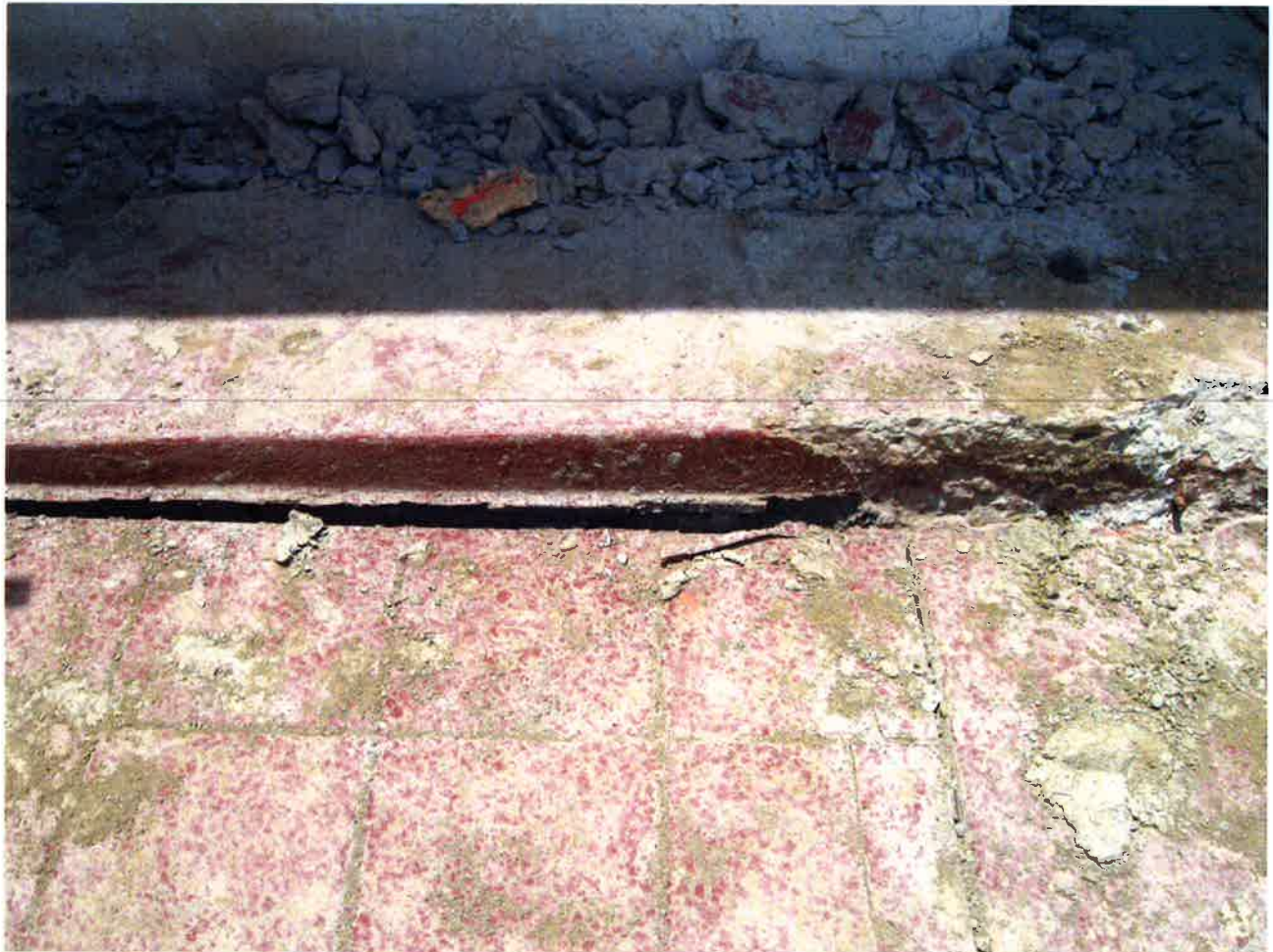
Figure 8: Core drilling from 2006 Pressure Grouting resulted in destroyed patio slabs
