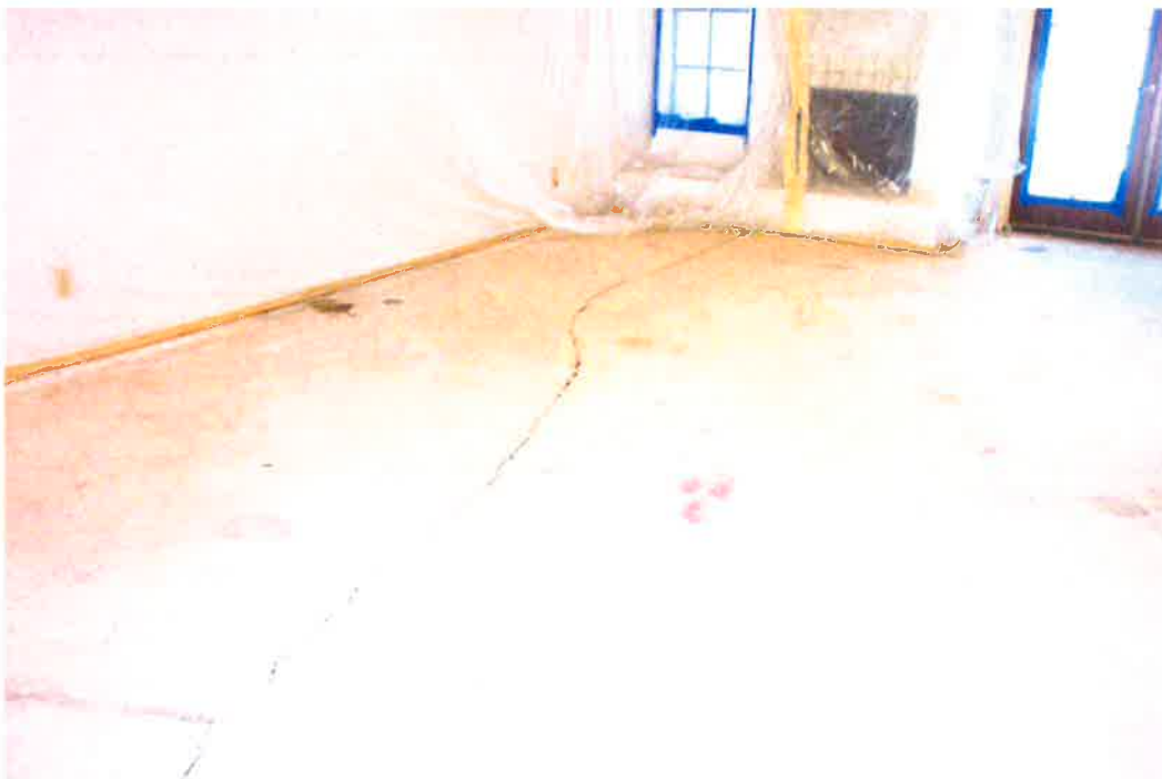
Figure 16: Slab cracking and damage as a result of ground settling
