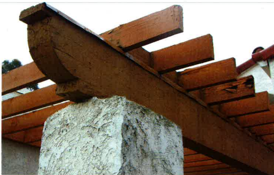
Figure 63: Termite and dry rot damage to arbor and support column
