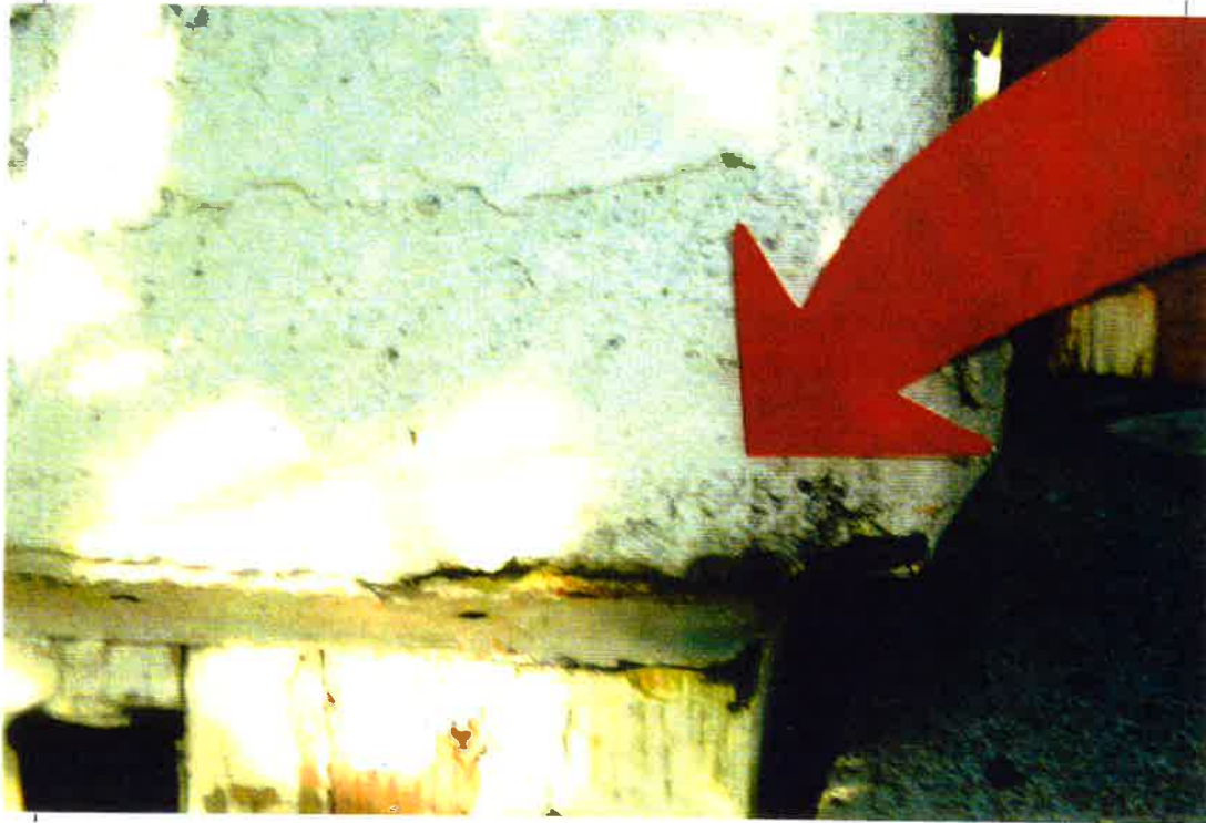
Figure 27: Rotten fence base and stucco
