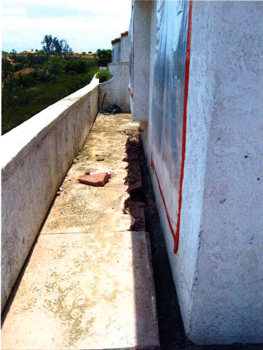
Figure 11: Core drilling from 2006 Pressure Grouting resulted in destroyed patio slabs
