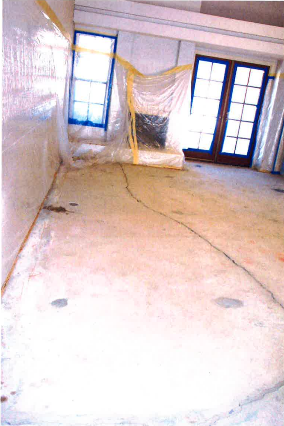
Figure 17: Slab cracking and damage as a result of ground settling
