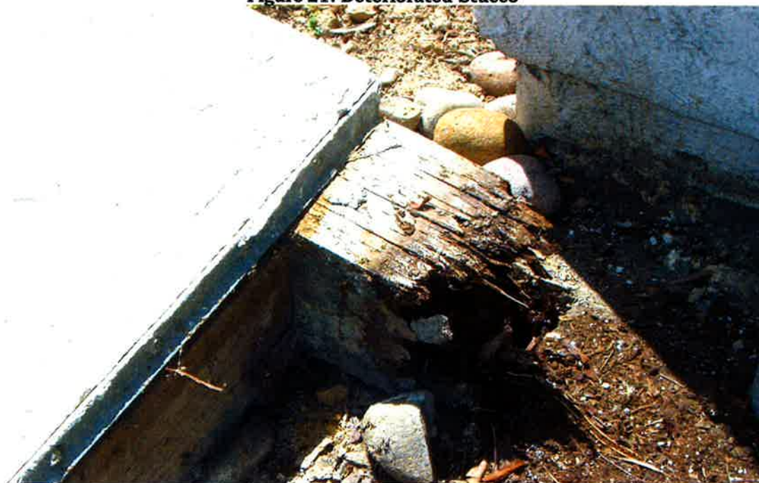
Figure 22: Rotted Wall Post
