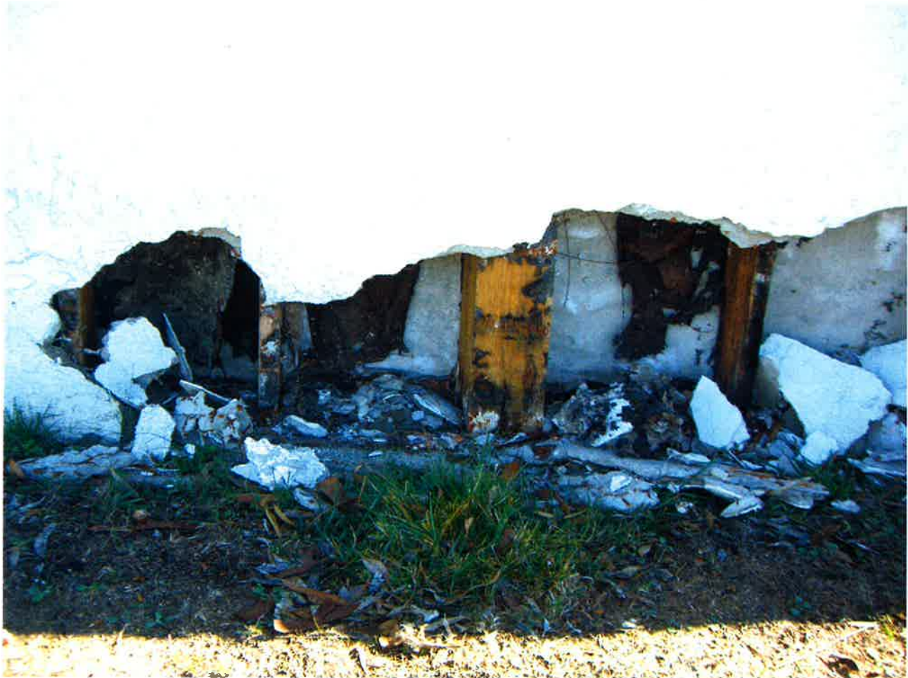
Figure 46: Garden wall. Note disintegrated black paper due to sustained dampness
