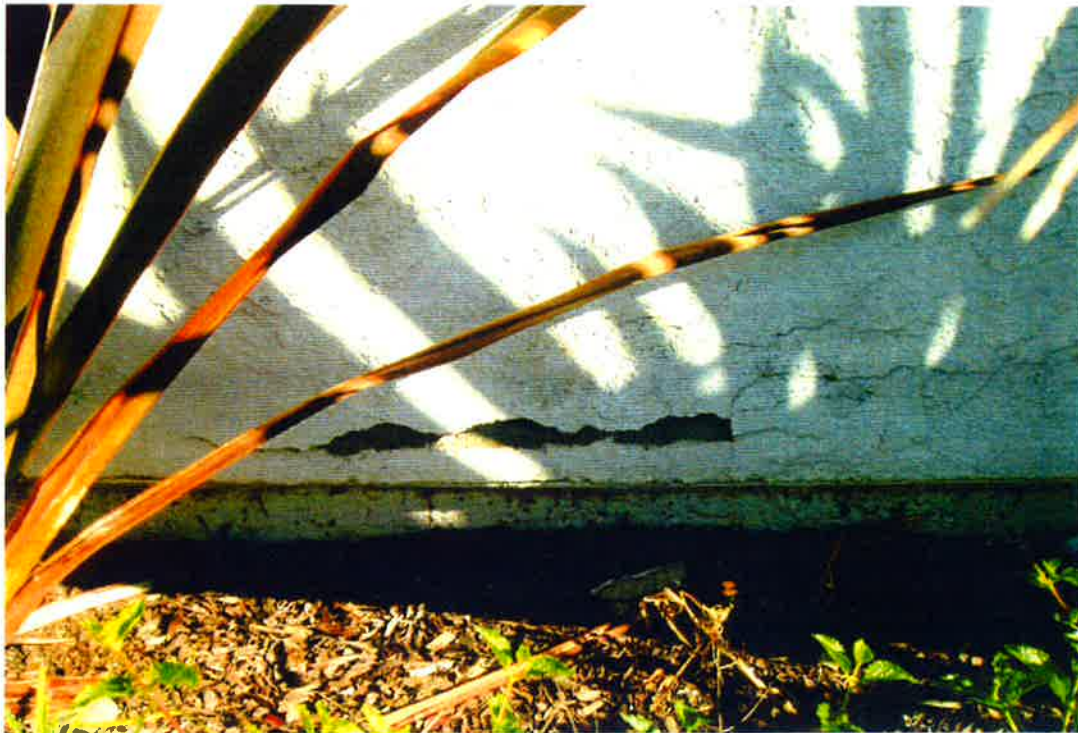
Figure 34: Stucco failure - sustained moisture
