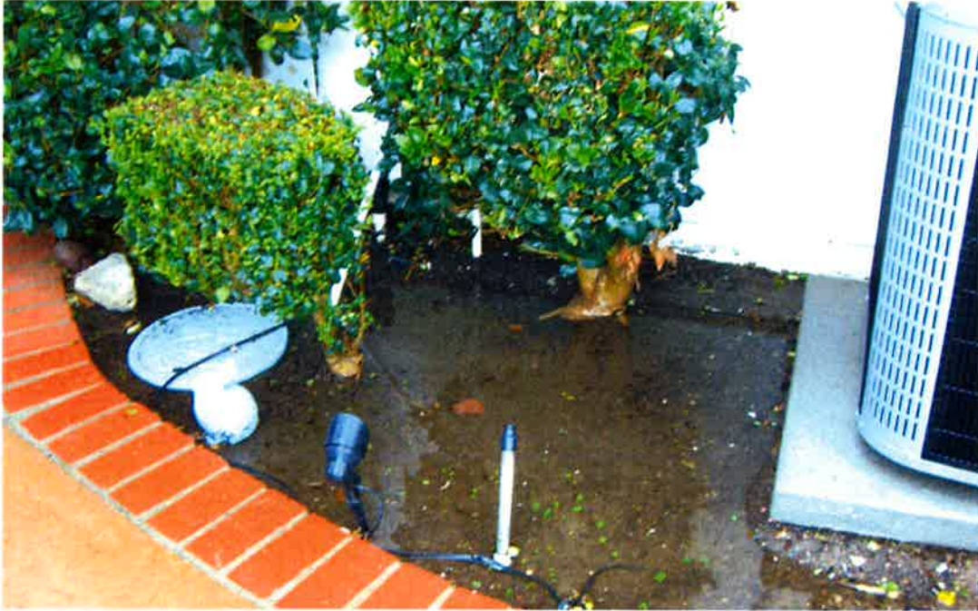
Figure 42: Water “ponding”, unable to drain away from house
