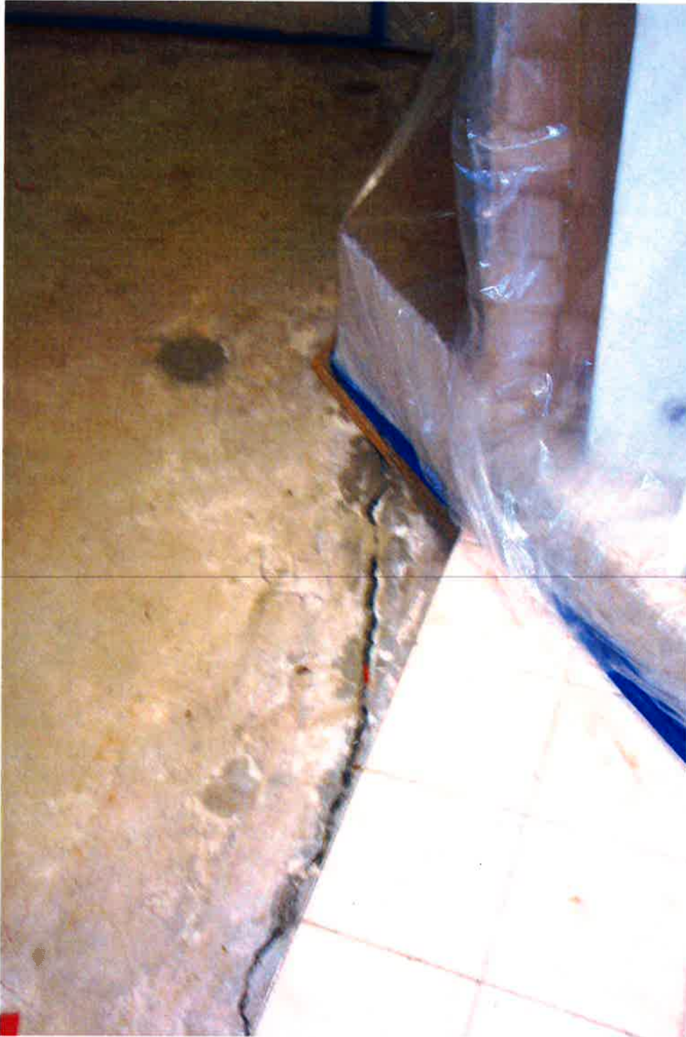
Figure 2: Slab cracking and damage as a result of ground settling
