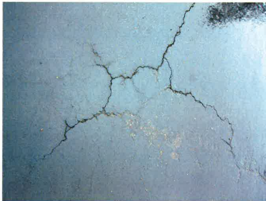
Figure 75: Cracks allow moisture, causing additional damage
