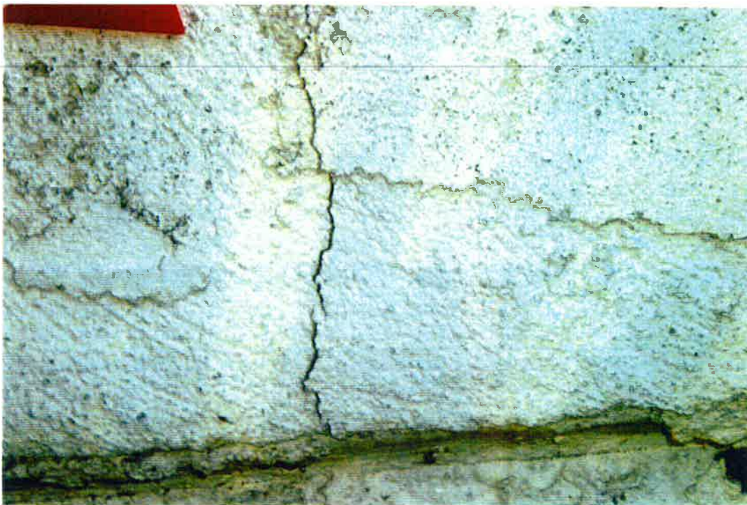
Figure 38: Cracked stucco due to ground shifting
