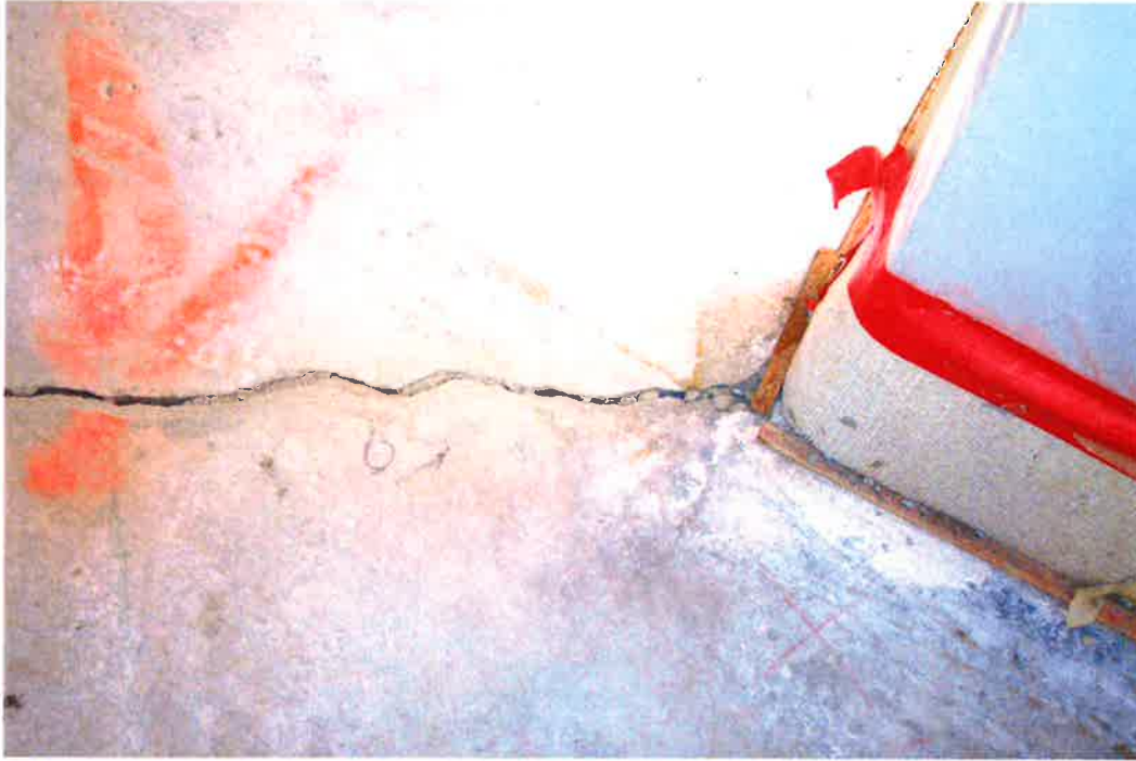
Figure 18: Slab cracking and damage as a result of ground settling
