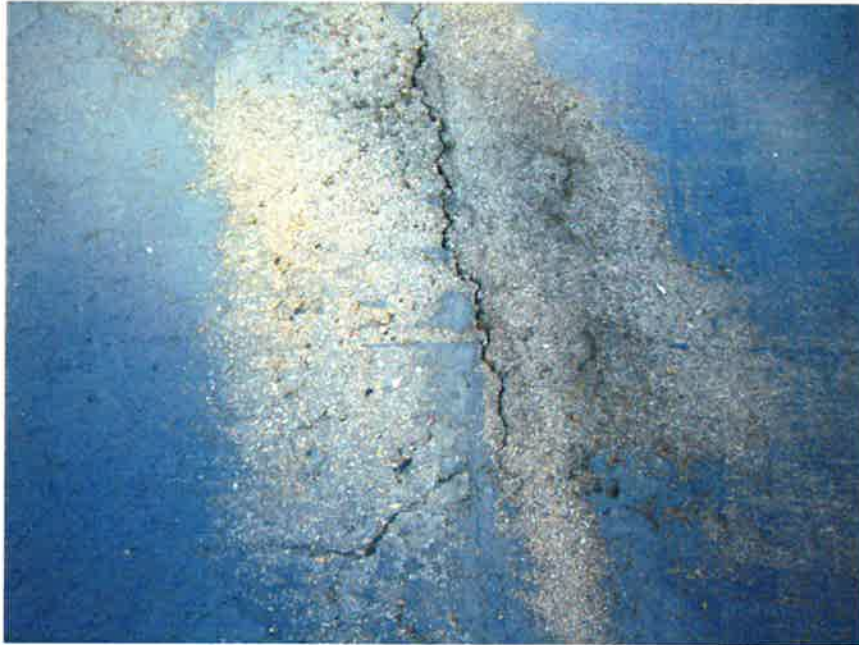
Figure 76: Breaks in surface allow moisture in causing additional damage
