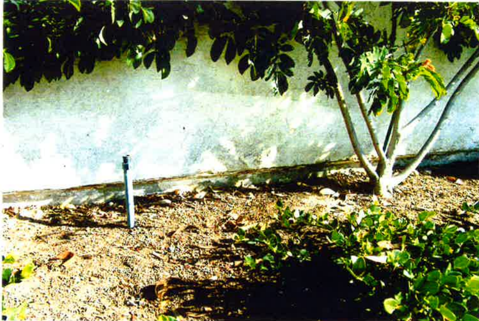
Figure 33: Stucco failure - sustained moisture
