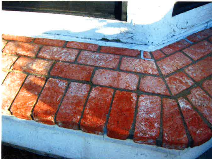
Figure 67: Crack at juncture of the Pot Shelf and building allows water intrusion
