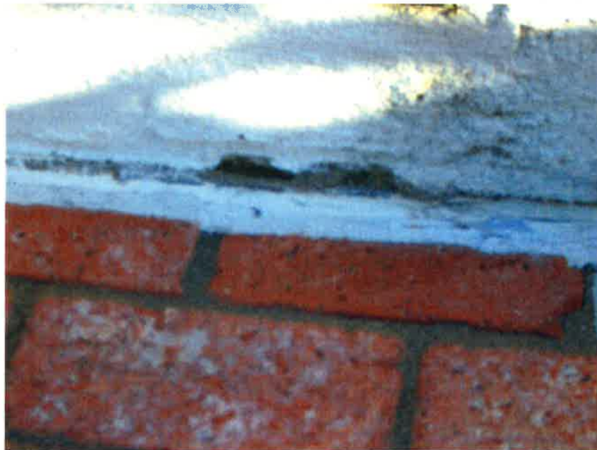
Figure 68: Close-up of crack between Pot Shelf and building wall
