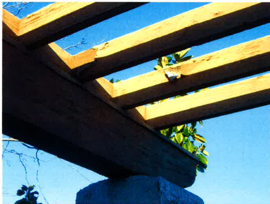
Figure 73: Peeling of and weather damaged paint
