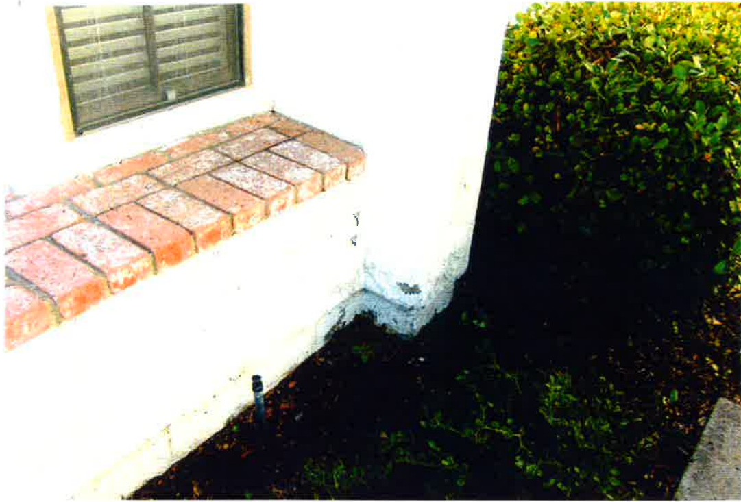
Figure 70: Inverse drainage, stucco and pot shelf failure
