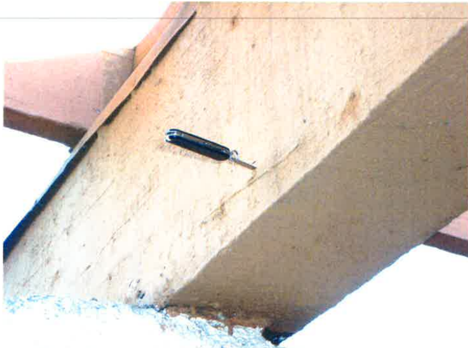
Figure 59: Knife easily penetrates arbors due to termite and dry rot damage
