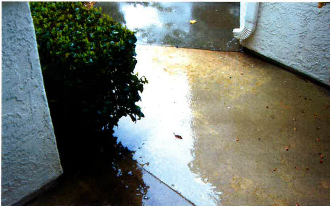
Figure 43: Rainwater “ponding”, unable to drain away from house
