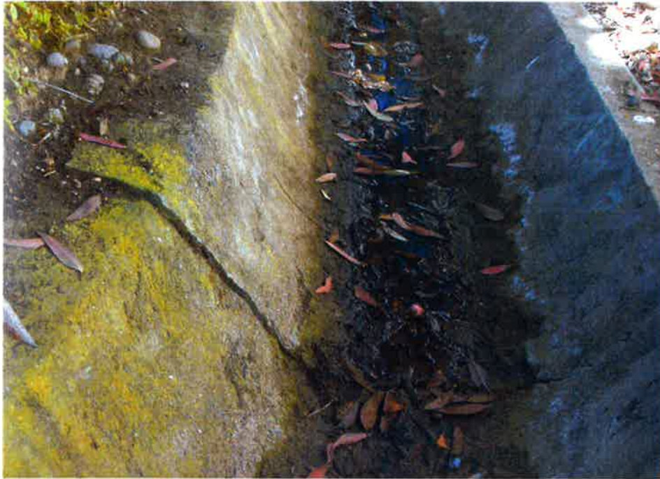
Figure 5: Damaged by shifting slope
