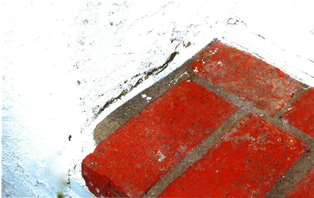
Figure 66: Crack at juncture of the Pot Shelf and building allows water intrusion
