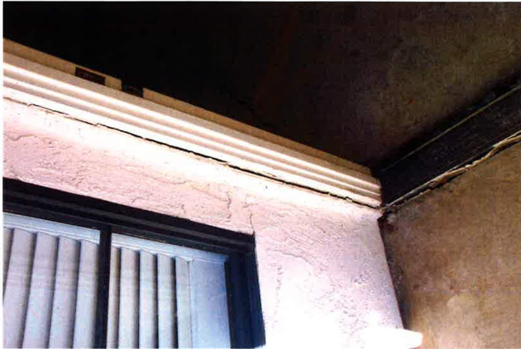
Figure 15: Wall separation from Pressure Grouting re-leveling of building
