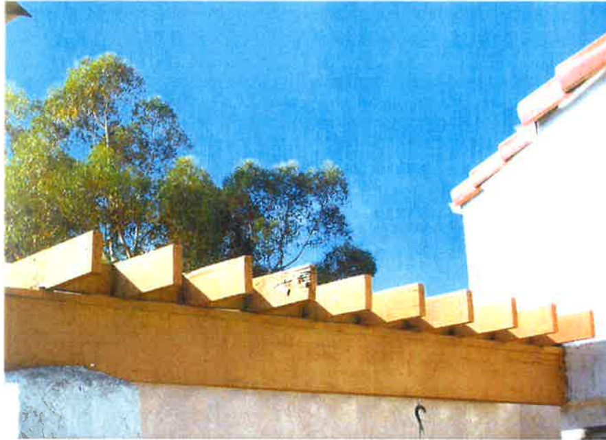
Figure 64: Termite and dry rot damage
