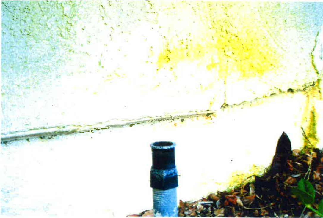
Figure 39: Sprinkler location and stucco failure
