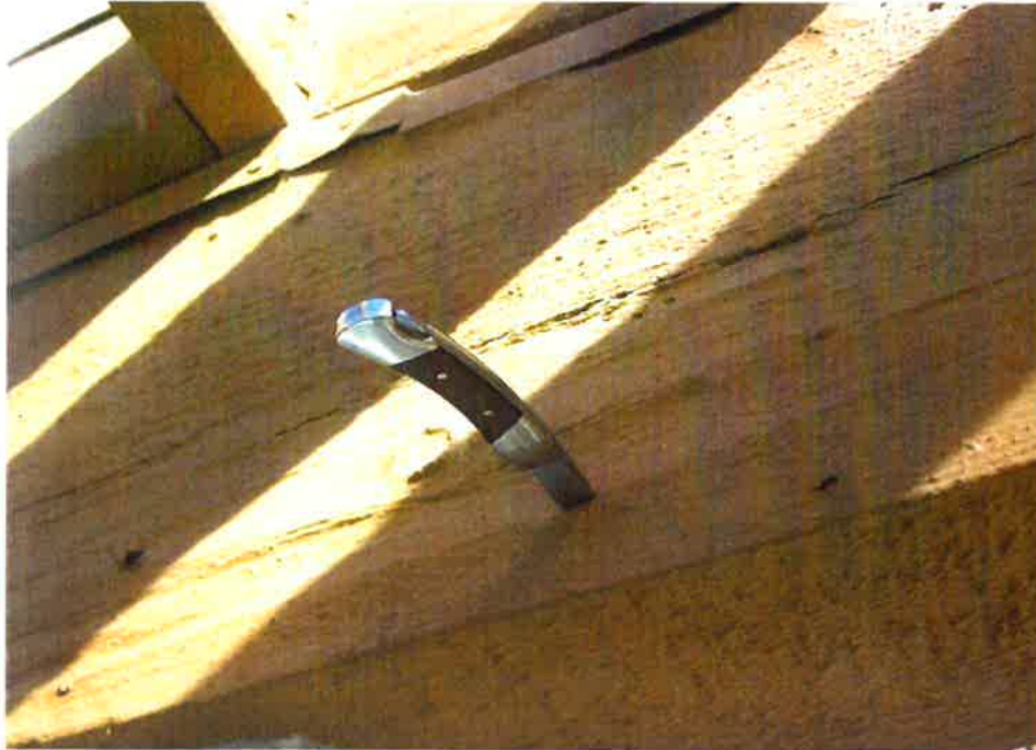
Figure 60: Knife easily penetrates arbors due to termite and dry rot damage
