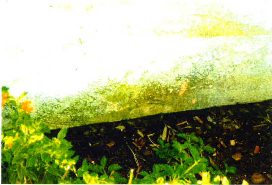
Figure 35: Stucco failure – sustained moisture
